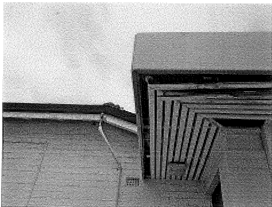
Part of the west wall: original roads board building (left) and 1964 addition (right).
