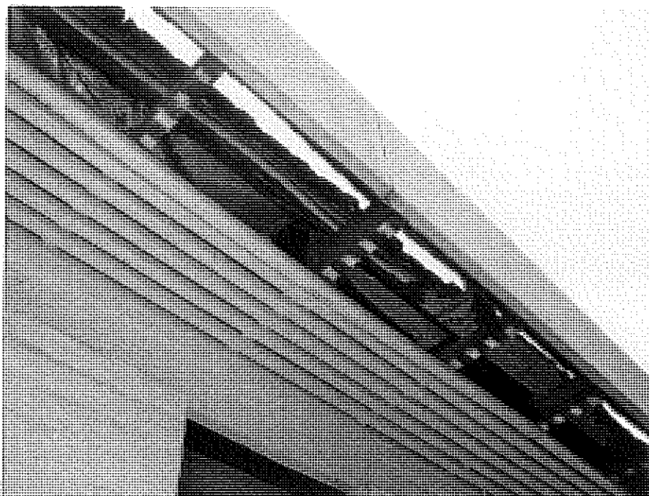
Eaves and box gutter detail along the south wall of the 1964 addition.
