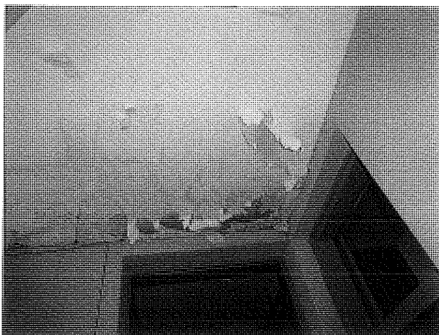
Interior: ceiling that is part of the 1964 addition- typical of the ceiling condition throughout of that addition.
