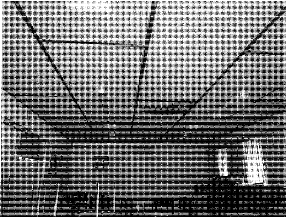
Interior: ceiling in the Council Chamber of the 1964 addition showing water damage.
