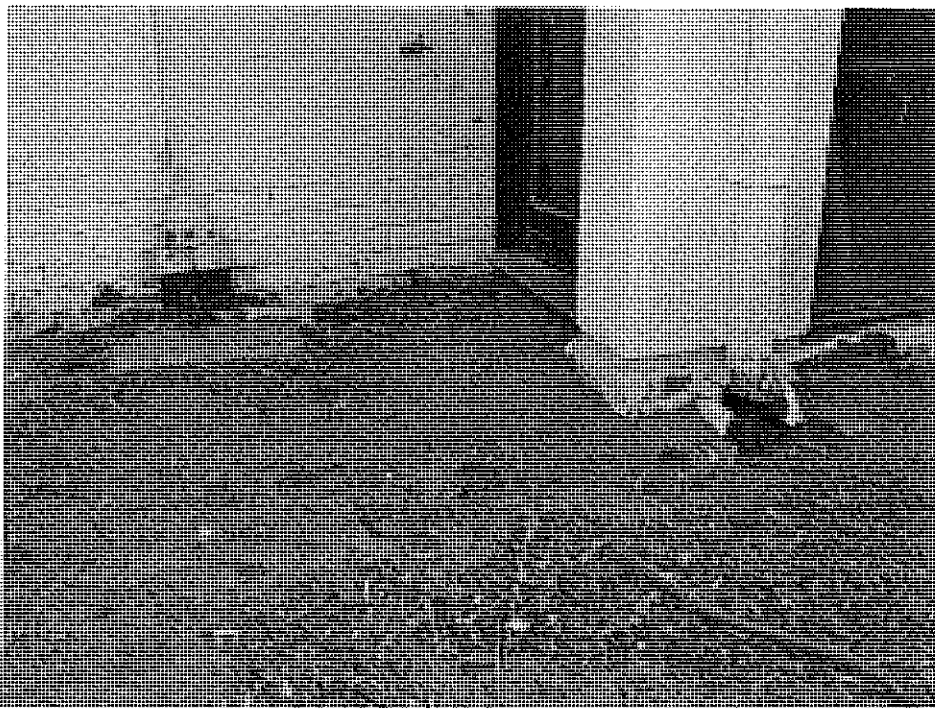
Part of the west wall: original roads board building (left) and 1964 addition (right) showing the ground level drainage issues.
